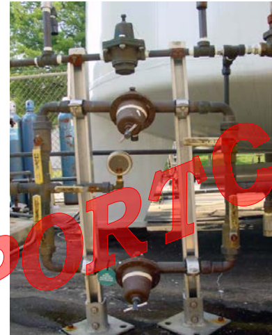
HOSPITAL'S GAS SUPPLY SOURCE
